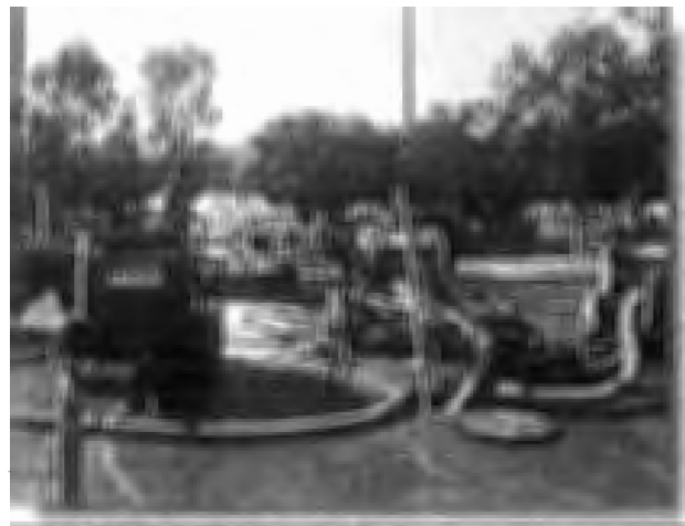
Figure 2-8 Typical Sewer Bypass Pump Setup
