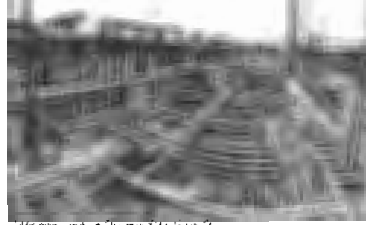
Wastewater Pump Station 2 Reliability Upgrades & Power Generation System City of San Diego
